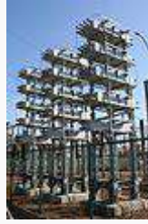
75MVAR substation capacitor bank at 150kV
